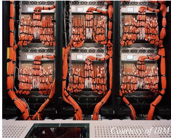
Figure 2.9: IBM MareNostrum central switch rack, with 1700 fiber cables/rack
